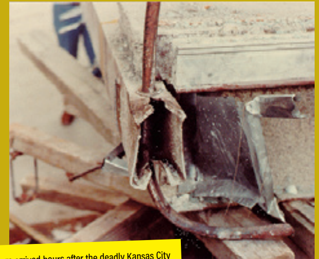
ON THE SCENE WJE investigators arrived hours after the deadly Kansas City Hyatt Hotel walkway collapse in 1981 to inspect the collapsed structures.
