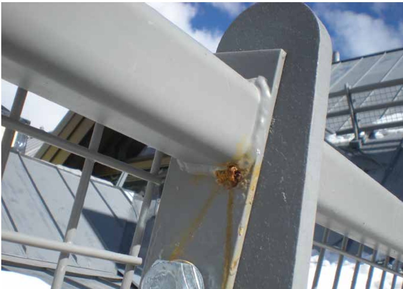
Figure 3. Rust stain appeared to originate on most affected samples from a ¼-inch spot at the corner of the weld.
