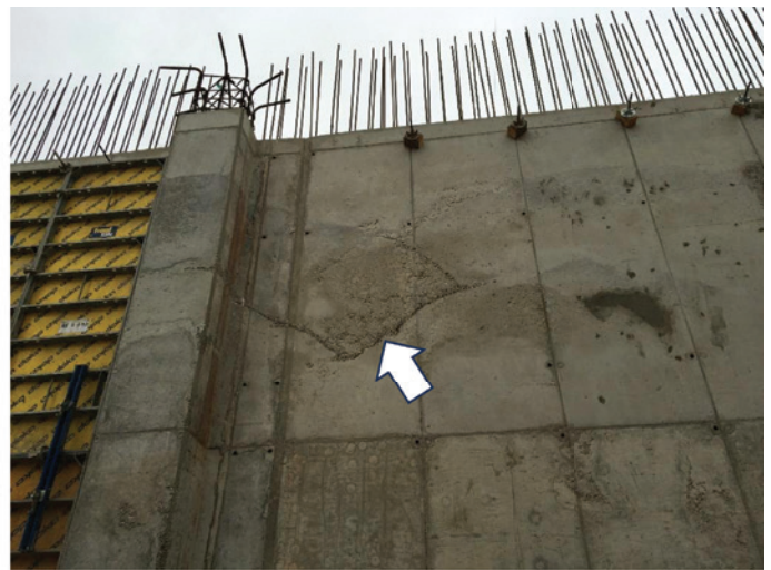
Figure 9. Honeycombing on surface of blast wall (marked with arrow).
