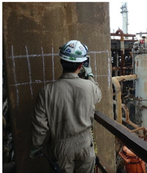
Figure 1. GPR survey being performed to locate reinforcing steel in a column as part of a structural evaluation in a refinery.
