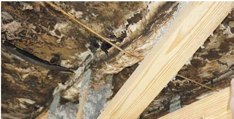
Figure 1. Sheathing and truss failure in insulated roof framing system (insulation removed to show distress).
