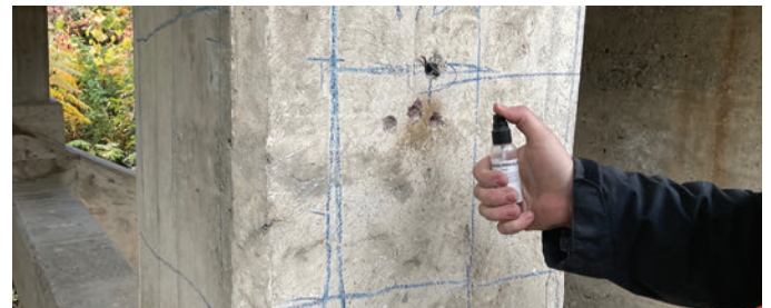
Fig. 8a: Carbonation Field Test—spray-applied pH indicator (phenolphthalein) at drill holes of incremental depths
