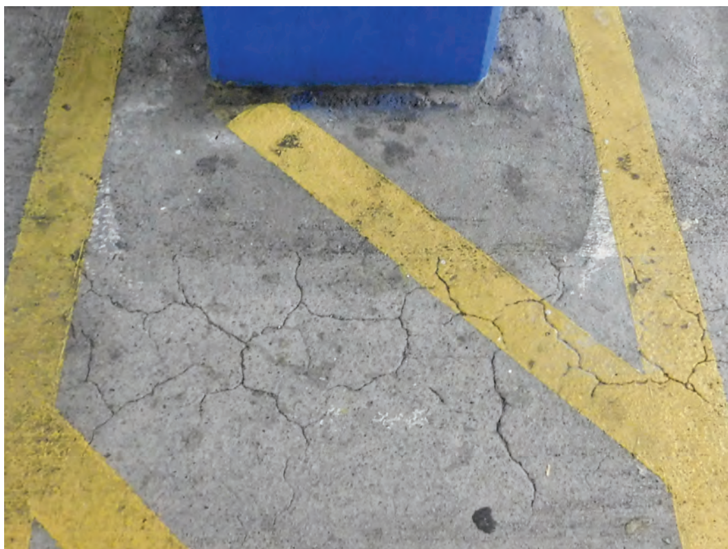
Fig. 5. This photo shows a swath of slab that has been bead-blasted or otherwise ground down to remove a curved white line; the mechanical removal of the line resulted in the cracks that were already present in the slab becoming noticeable due rounding of their edges.
