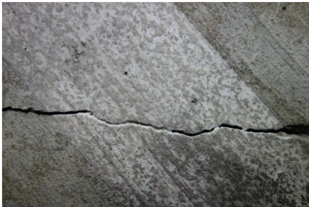
Fig. 4. Paint from this parking stall stripe is present within and spanning across the crack, indicating that the crack was present at the time the paint was installed and that the crack has not moved substantively since.
