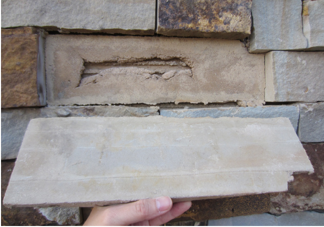
Figure 5. Void in Adhesive Mortar
